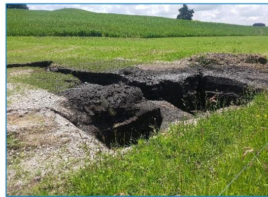
Image 2: Damage from eroded EFP
